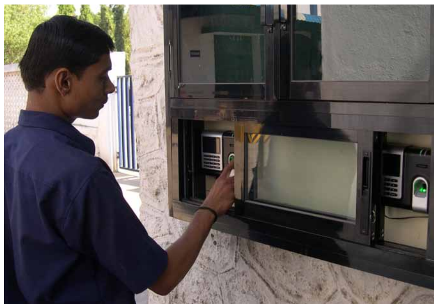
Biometric finger print scanning systems have been installed at the offices and factories to control access to the facilities
